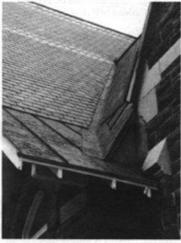
This photograph shows the flashing for an open valley where two roofs meet. The width of the valley increases as it approaches the eaves in order to accommodate the increased flow of water.
