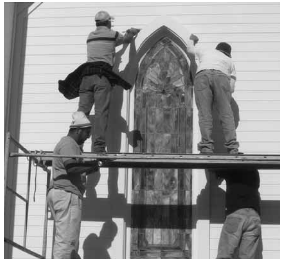
A crew installs a stained glass window at Discovery UMC's new location, one of several windows restored by Central Texas artisans.
