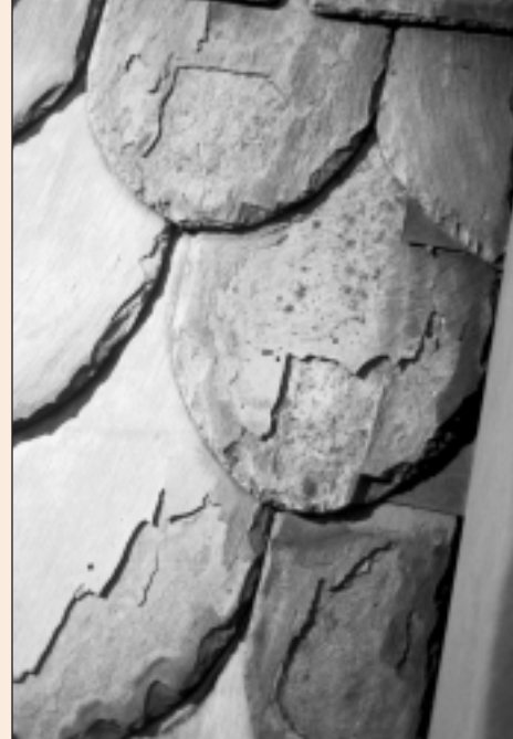
Pennsylvania black fish-scale slate on a church rectory in Philadelphia shows obvious evidence of delaminating.
