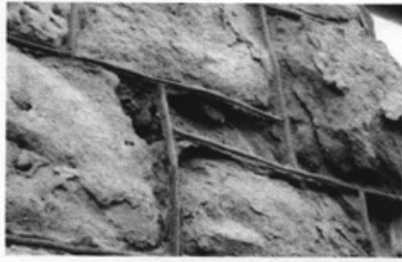
In this dramatic example of the effects of hard repointing mortar on a Brooklyn church, the much softer, porous stone has spalled and eroded, leaving the impermeable mortar in place.
