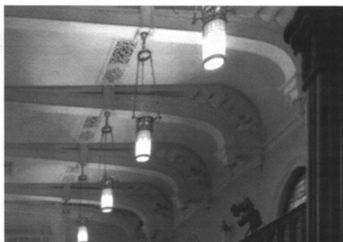
The sanctuary of St. Stephen's Episcopal Church, 10th Street below Market Street, is equipped with ornate grilles that run in parallel rows like this one along the ceiling. This system, which has been used since the 1920s to ventilate the building, may be used by the congregation in the near future to implement central air-conditioning. Detail of photo: William Douds Photography.
