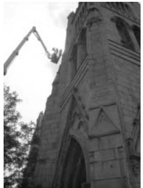
Atkin Olshin Schade works on Philadelphia Fund grantee Arch Street United Methodist Church.
