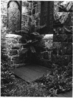
The tenacious Ailanthus , or Tree-of-Heaven weed can thrive in foundation cracks.
