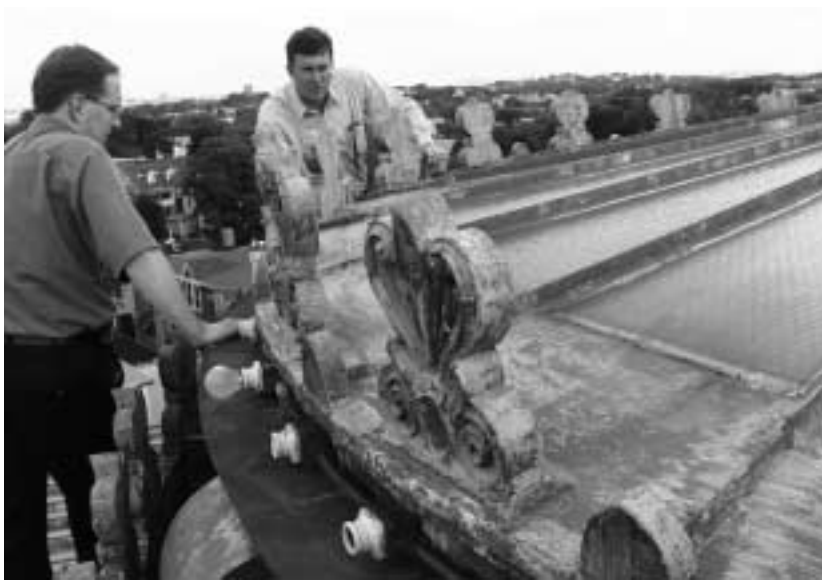
HBI Steeples Project grantee Second Church of Christ, Scientist in Roxbury, MA, gets a roof inspection.
